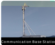
Communication Base Station
