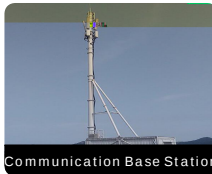
Communication Base Station
